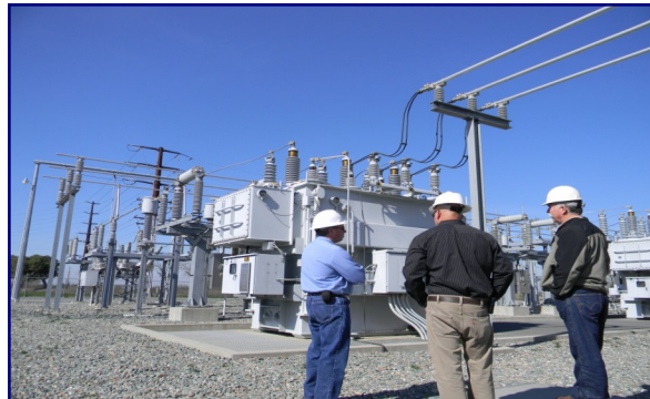
An MID electrical technician, manager and safety supervisor examine a transformer at a Merced-area substation.
