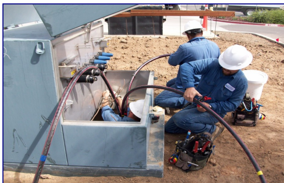
A crew from MID's Energy Services Department connects power to Mercy Medical Center Merced's new hospital in North Merced.
