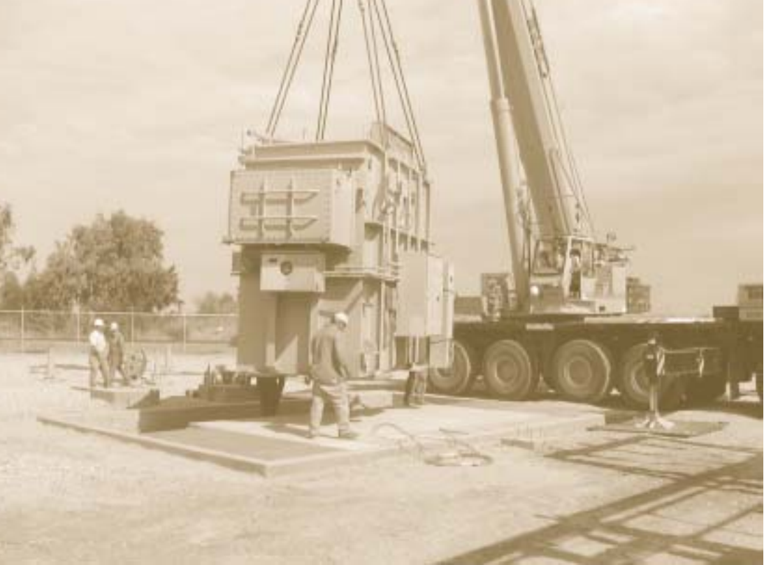
NEW TRANSFORMER INCREASES POWER CAPACITY AND FURTHER IMPROVES SYSTEM RELIABILITY.
